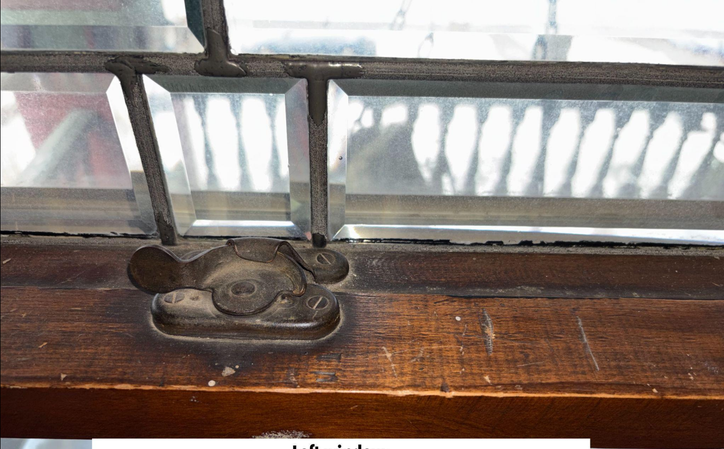
Left window: Dowel indentations from weight of window on top of lower sash. White powder lead dust from soldering corrosion.
